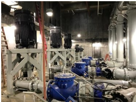
Figure 2 —Wastewater Pump Station (Photo provided by: P. Hubbard, HRSD)
